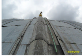
242. Lead sheets lifted & misaligned
