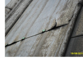
251. lead sheet tear on SE face
