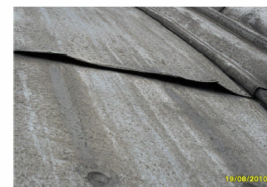
249. Leadwork tearing @S
