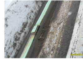
247. Old soldered fixing failed @SE
