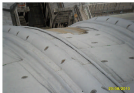
252a. Lead staining & missing section
