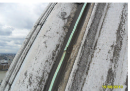
246. Descent 3 loose copper cleat & downtape @SE
