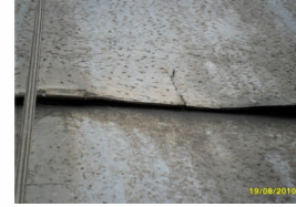
250. Vertical crack up lead sheet S face
