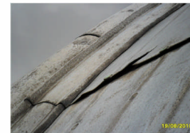
252. Lead sheet tear
