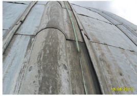
241. Lead sheets misaligned @ SW
