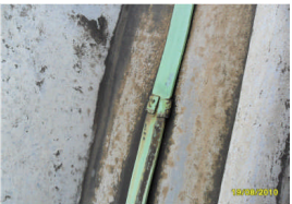
245. Descent 3 loose copper cleat SE downtape Descent 3
