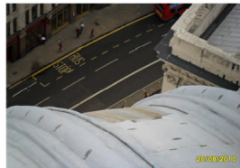
252b. Lead staining & missing section @ SW
