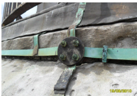
243. Golden Gallery Base LC coronal conductor tape & fittings attached @SE
